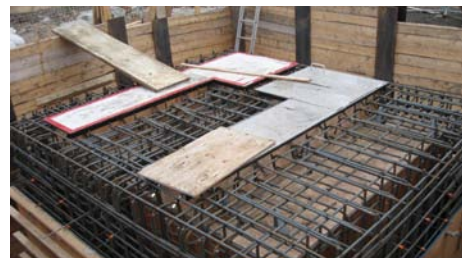
The overflow chamber in progress: the walls are seven metres high and 16 inches thick.
